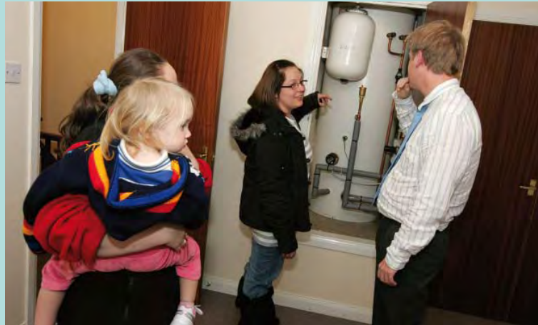
Residents in Hook, Hampshire, discuss their ground source heat pump installation with a TVH staff member
